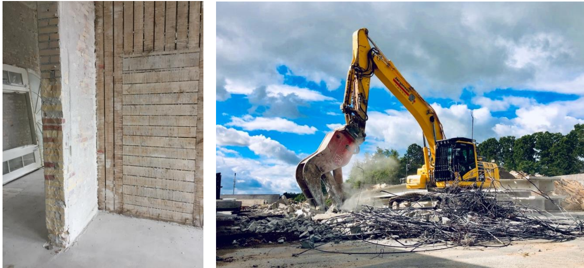
Figure 7 Surface covering is removed from walls and floors prior to further demolition and deconstruction (to the left), reinforced concrete is separated into concrete and metal fractions on site (to the right) (Source: Danish Technological Institute)
